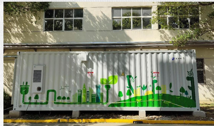
Location: Vietnam Configuration: Energy storage Scale: 400kW/1.6MWh Result: Successful acceptance
