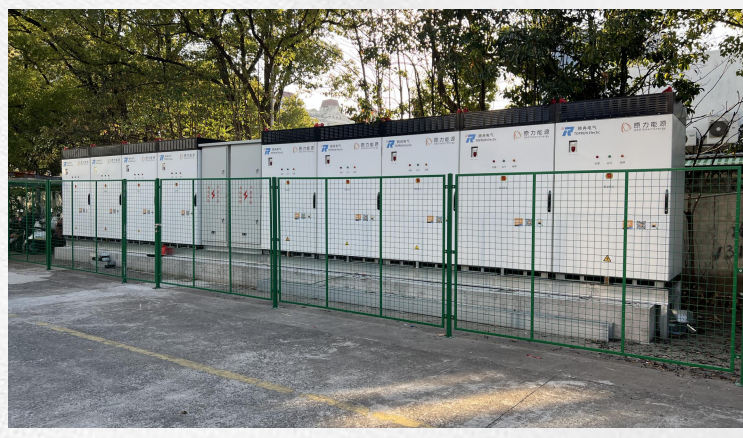
Location: Shanghai, China Configuration: Energy storage Scale: 3MW/6.45MWh Result: Successful acceptance
