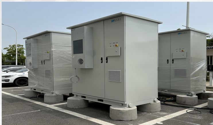
Location: South Africa Configuration: Energy Storage Scale: 300kW/645kWh Result: Successful acceptance
