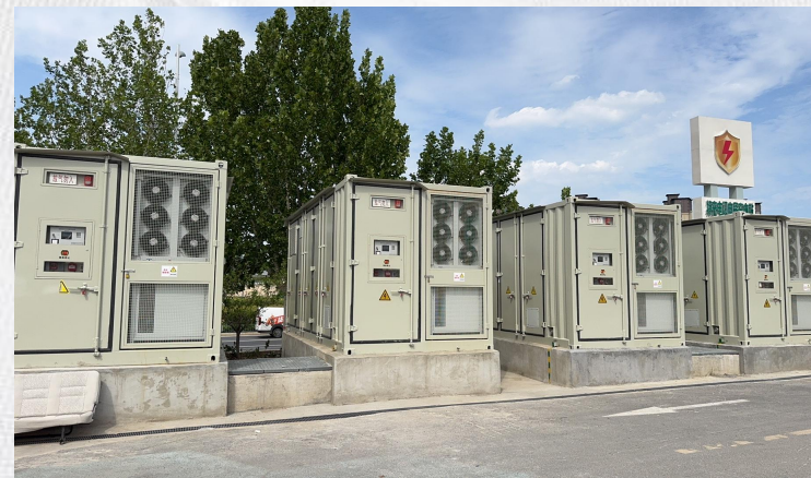
Location: Henan, China Configuration: Energy Storage Scale: 6.9MW/11MWh Result: Successful acceptance
