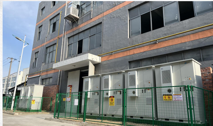
Location: Suzhou, China Configuration: Energy storage Scale: 600kW/1.2MWh Result: Successful acceptance
