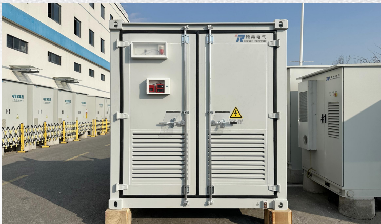
Location: Hong Kong, China Configuration: Energy storage Scale: 372kW/372kWh Result: Successful acceptance
