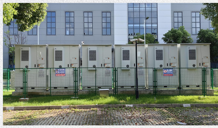
Location: Suzhou, China Configuration: Energy storage Scale: 3.44MW/6.88MWh Result: Successful acceptance
